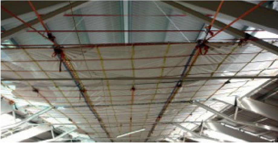
View from below the WalkAbout system.
